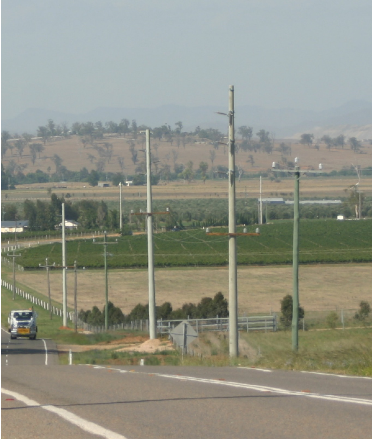
Figure 4.5a | The proposed transmission line will be similar to the one shown above with distribution lines located on a wooden cross bar with higher voltage transmission line above. See pole marked. This transmission line is located on Denman Road, Muswellbrook.
