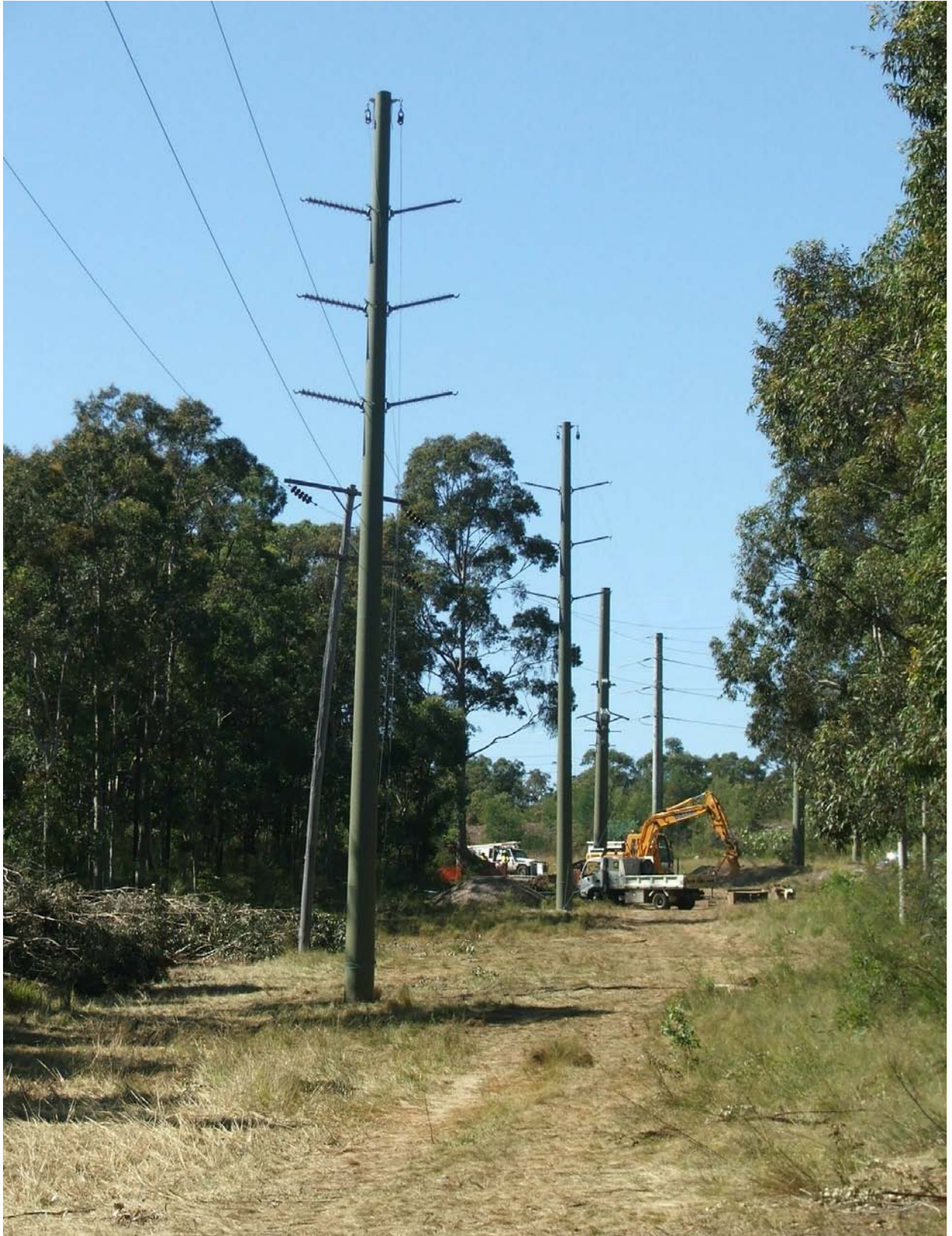
Figure 4.5b | This photo shows a single circuit 132kV transmission line. the proposed 66/33 kV line will have a set of insulators and conductors on both sides of the pole if option one is used. If option 2 is used there will only be one set of conductors as illustrated in the photo.
