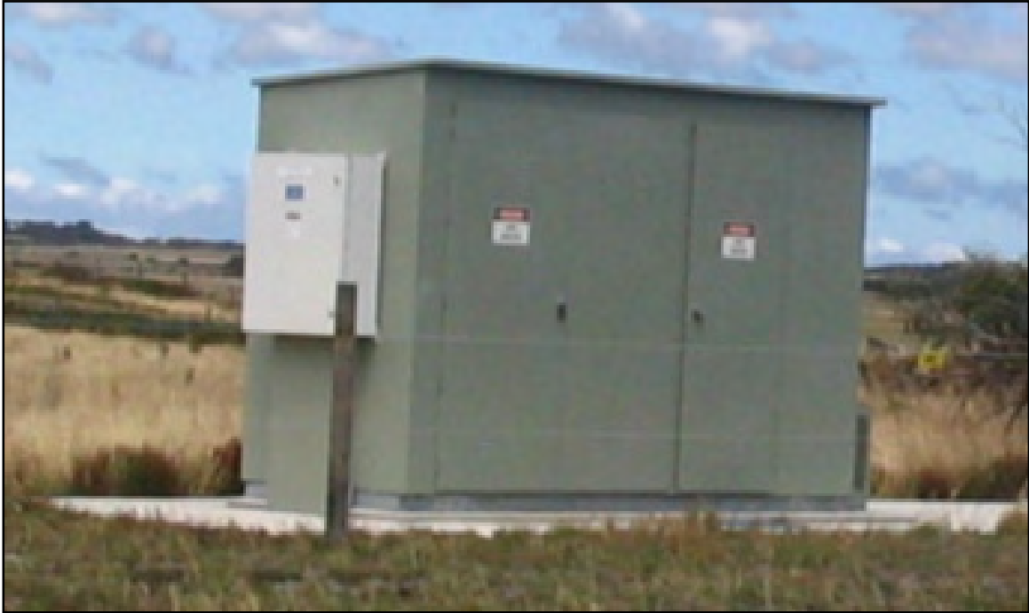
Figure 2.10 – PV Farm - Monitoring & Metering Cubicle (Econnect)
