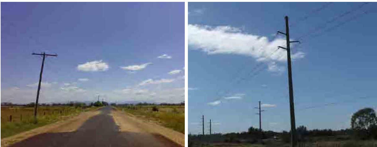
Photographs showing existing timber poles (left) and proposed replacement concrete poles (right) (Energy Australia 2007)
