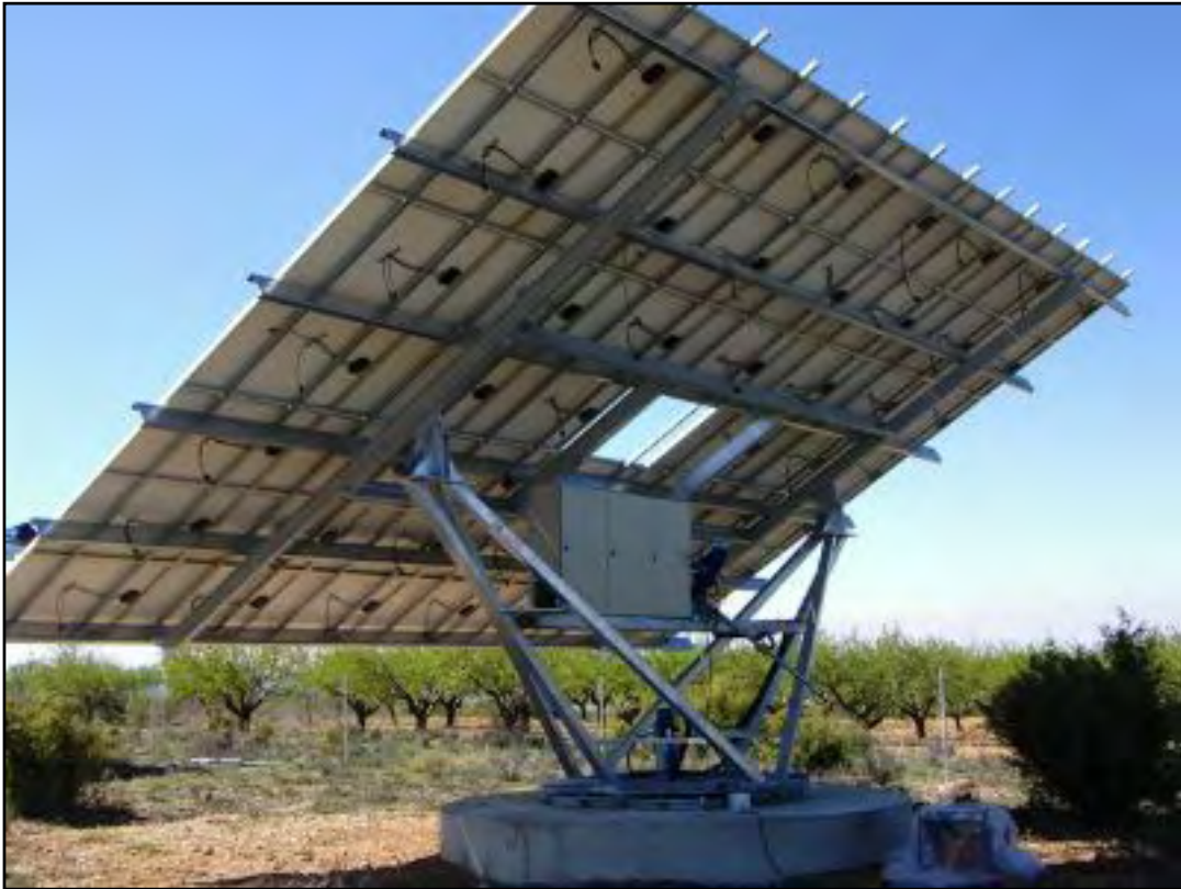
Figure 2.8 Solar PV Typical 11kW Dual-axis Tracker (Courtesy of Meca Solar Pty Ltd)
