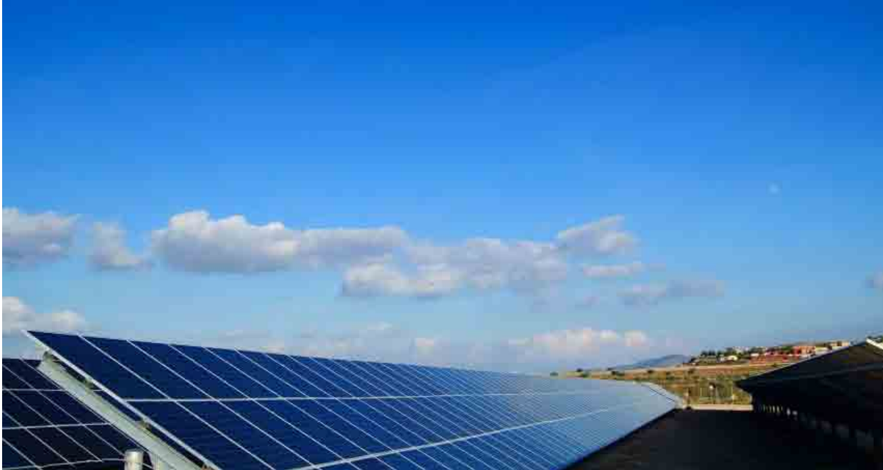
Image of a typical fixed- frame solar photovoltaic plant
