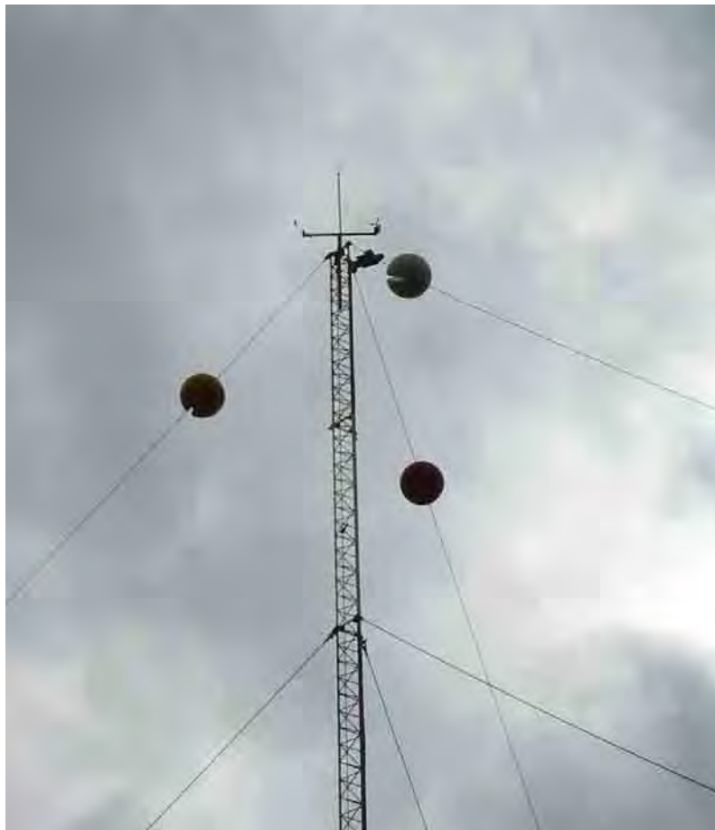
Figure 2.3 - Mounting of the anemometer and wind and wind vane installed at a height of 45m agl. A Data logger is installed closer to the base of the tower for logging ten minute mean wind speed and direction, standard deviation and maximum wind speeds.
